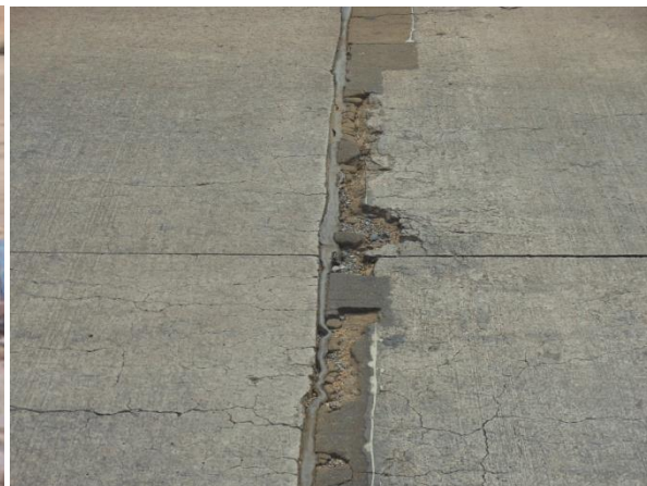
Photo 2: Spalled Transverse Joint
