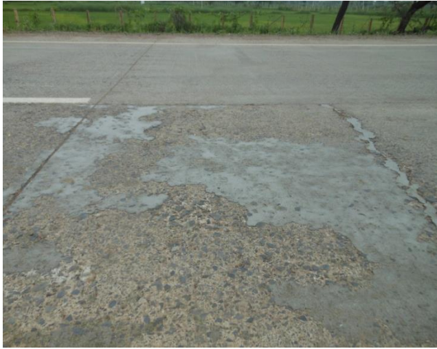
Photo 3: Abraded Concrete Surface
