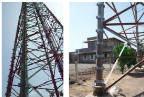
(i) Angular tower – Adding new main leg using dry clamps (ii) Hybrid tower (Main legs : Pipes) – Adding new flats with dry clamps
