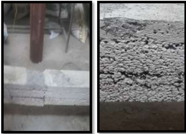
Fig –12: Impact Strength Test Cracks
