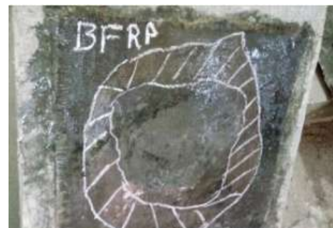
Fig 12: Failure pattern of BFRP wrapped rehabilitated slab
