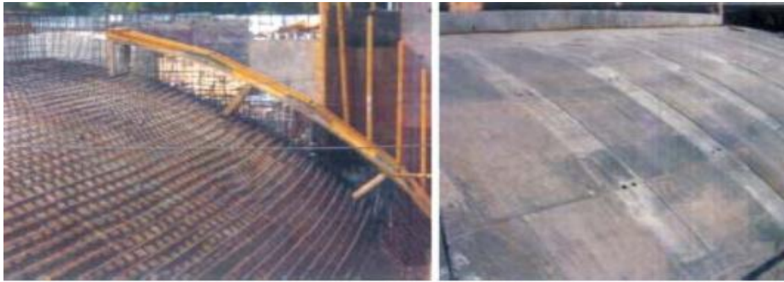
SCC poured at Rotary Dome at central secretariat station – Delhi Metro Project
