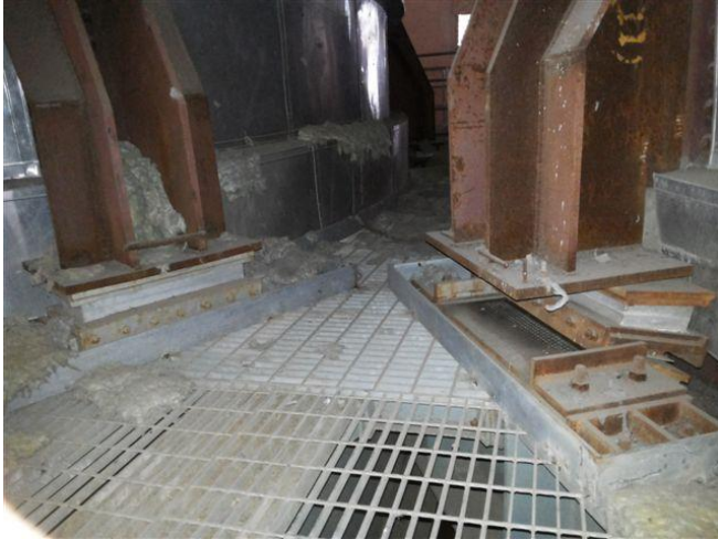
Exhibit-5- Dislodged bearing pad
