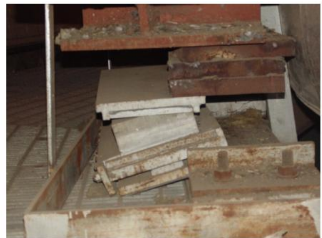
Exhibit-8- Dislodged bearing pad
