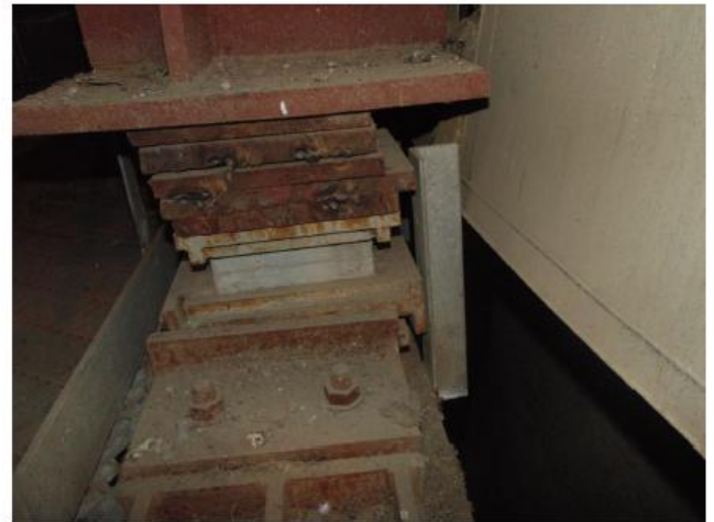
Exhibit-7- Too many shim plates over the bearing pad
