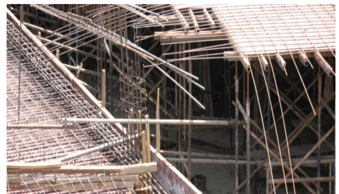
Fig 3 - Unplanned Construction Joints
