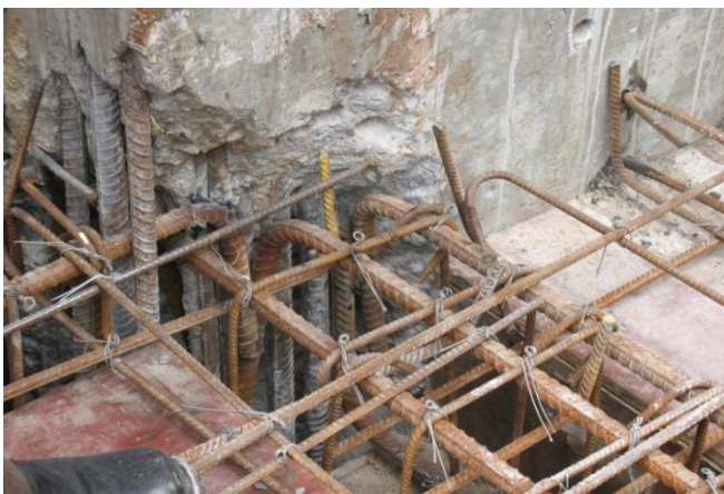
Fig - 1 Missing Dowels (1)
