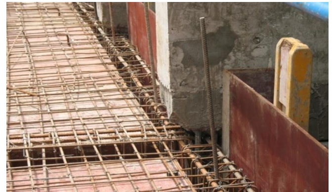
Fig - 2 Missing Dowels (2)
