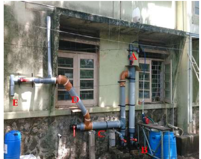
A – Inlet from roof top + Coagulation B – Drain Valve C- Horizontal Tube settler+ control valve D – Inclined Tube Settler E – Discharge Valve
