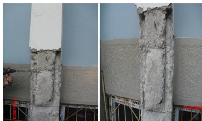
Fig.-4. Status of the columns
