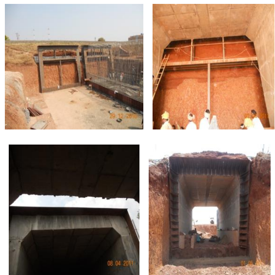
Fig 4: MS Plate/Front Shield for Box Pushing in RUB.
