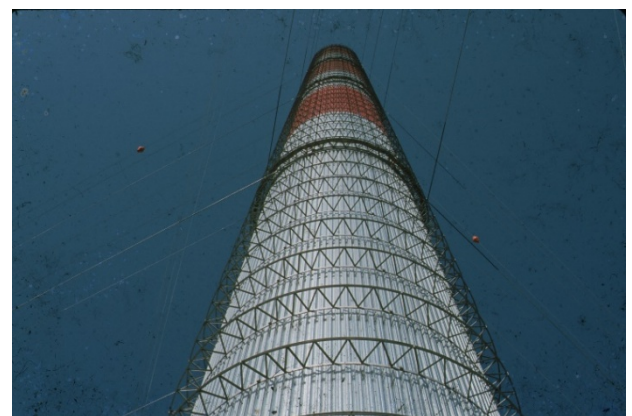
Fig -2: The Chimney in Manzaneres, Spain made of sheet steel rings supported by guyed wires
