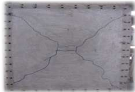
Fig 21 : Actual Crack on bottom surface for a Fixed Slab (Panel – 2) ( F_2 ) Subjected to UDL
