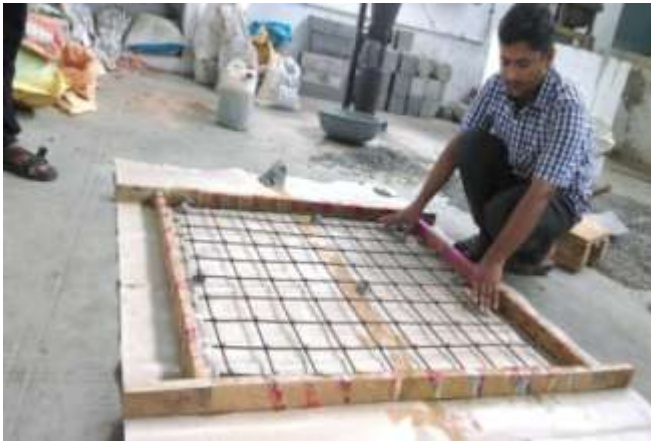
Fig.9: Shows the arrangement of reinforcement and clear cover blocks in GPC Slab
