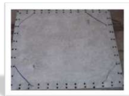
Fig 20 : Shows the Actual Crack on Top surface for a Fixed Slab (Panel – 1) ( F_1 ) Subjected to UDL
