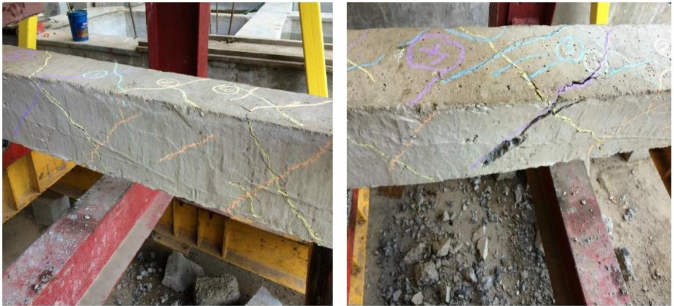
(a) Cracking Pattern in Beams
