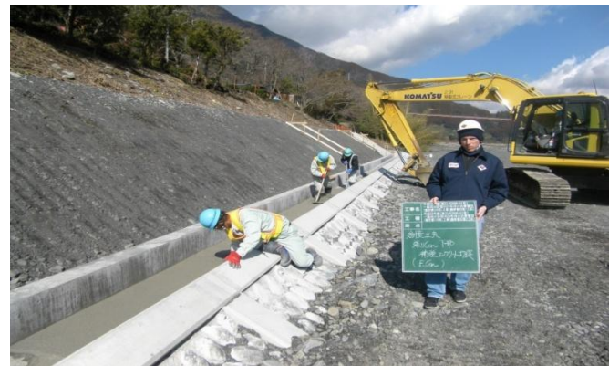
Fig. 9: Placement of Econ ® in Shizuoka area.
