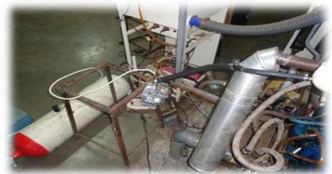
Fig.5. Natural gas cylinder, reducer and supply line
