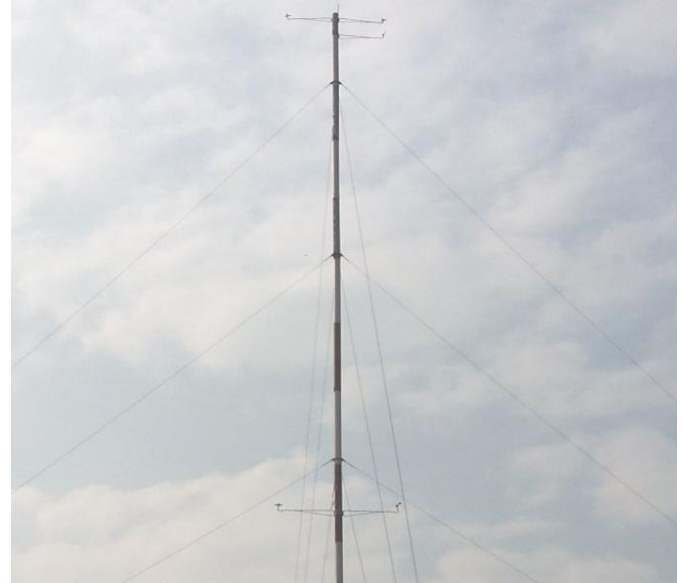
Fig 1- Wind mast at Energy Park, RGPV
