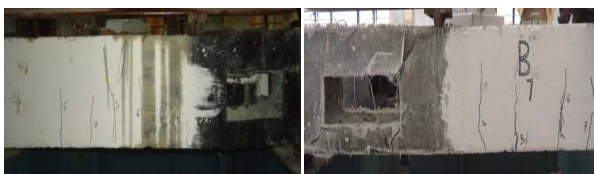
CFRP wrapping around the opening
