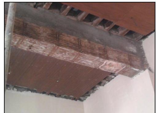
Fig -11: Longitudinally cracked beam with visible sag
