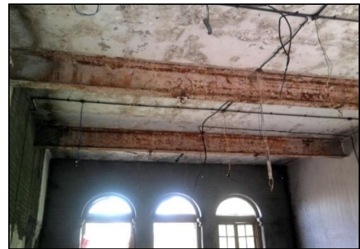
Fig -7: Corroded steel members due to leakage
