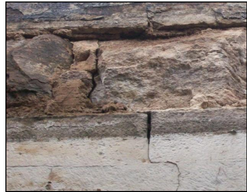
Fig -3: increased gap in joints due to growth of creepers
